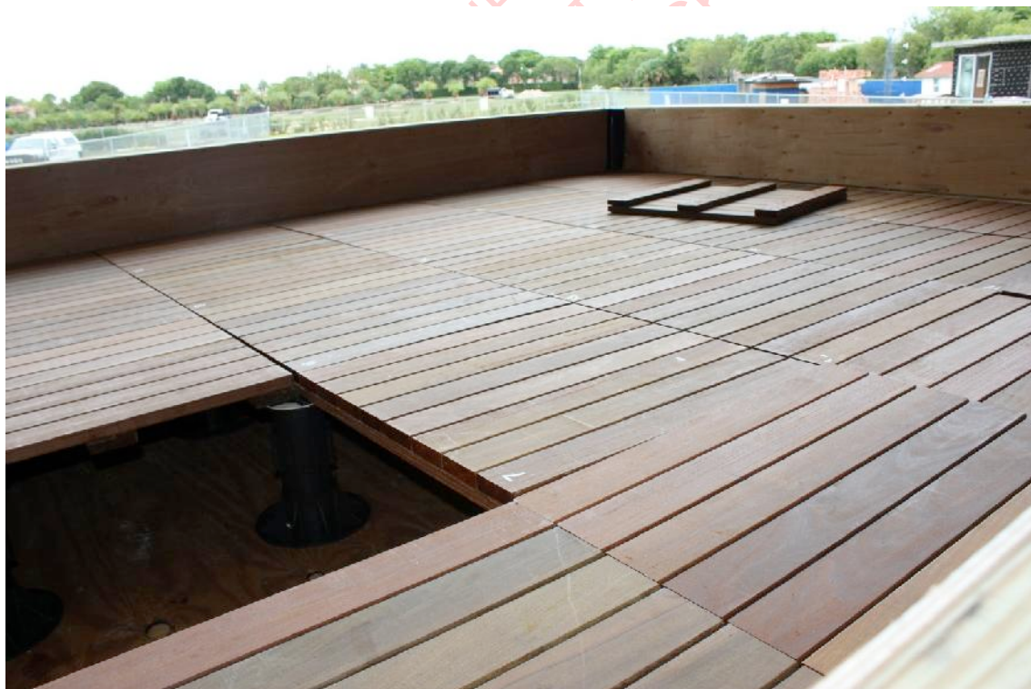
Figure 7 - Paver blown off into the leeward parapet
