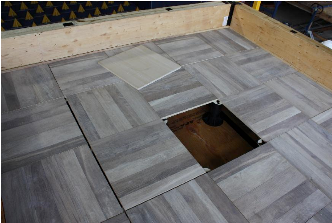
Figure 12 - Porcelain paver flipped upwards by the wind.
