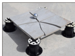
Broken paver supported by tray
